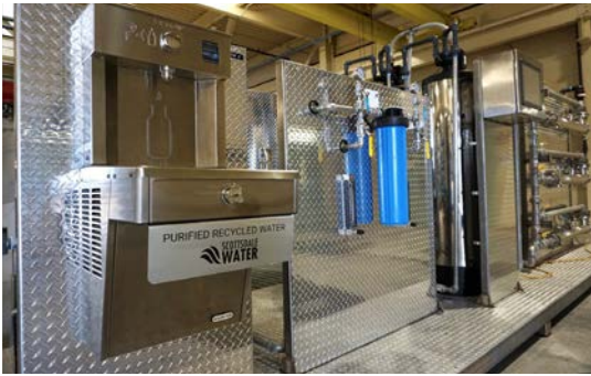
Purified Drinking Water demonstration station
