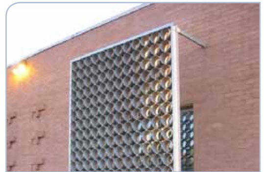
Sun screens can be incorporated into building architecture to reduce heat absorption.
